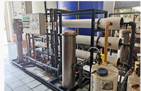
Reuse of wastewater by RO system TRJ (China)
