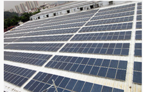
Solar panels installed on the roof, TRIN (India)
