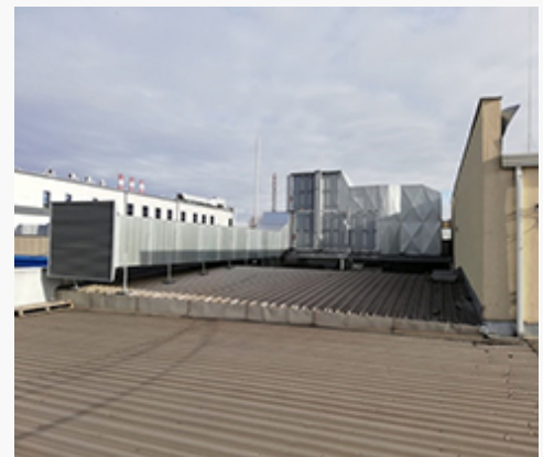
Appearance of equipment SRK-P (Poland)
