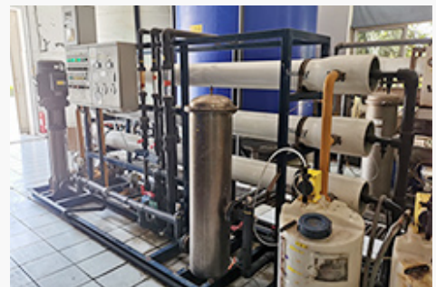
Reuse of wastewater treated by a reverse osmosis membrane system, TRJ (China)
