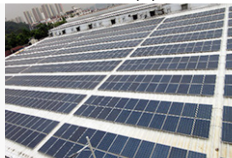
Solar panels installed on the roof, TRIN (India)
