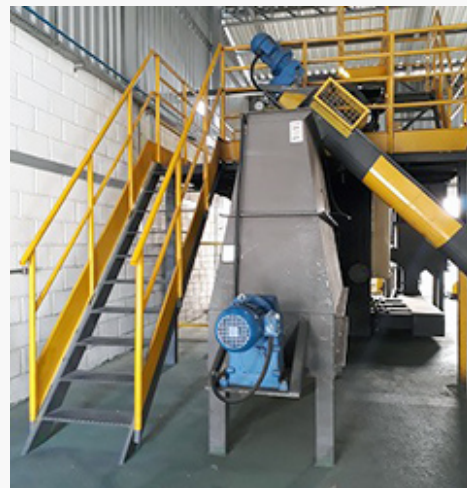
Newly installed wood-fired boiler, SRK-BI (Brazil)
