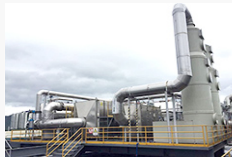
Equipment for treatment of gases generated by vulcanization, TRG (China)
