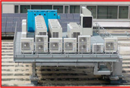
Outdoor units on the roof of old R&D headquarters
