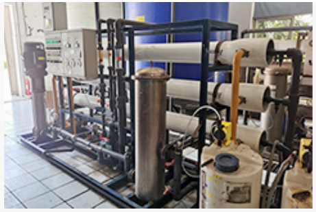
Reuse of wastewater by RO system TRJ (China)
